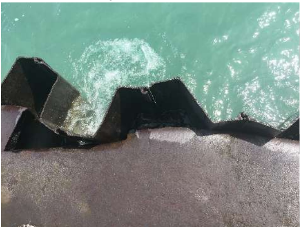
C. Bent/Broken Sheetpile Connections & Box
