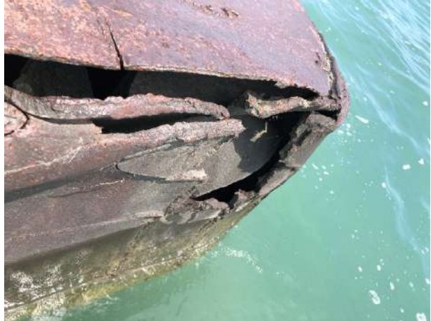
B. Damage to SE Outside Corner
