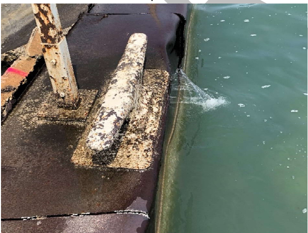
E. Water Escaping through Cracks in Box
