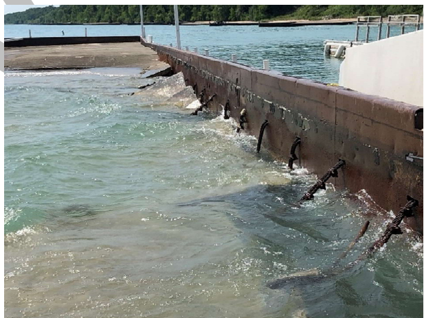
F. Broken Wire Rope Supports
