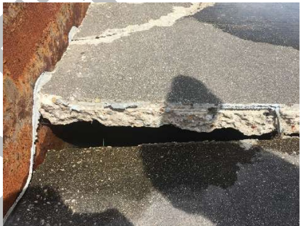
D. Concrete Slab Failure, 5" Thick
