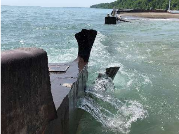
A. Broken Cargo Box Wall
