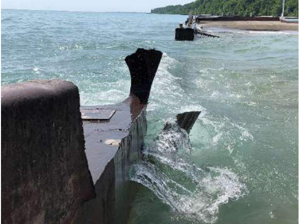
A. Broken Cargo Box Wall
