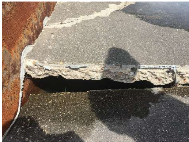
D. Concrete Slab Failure, 5" Thick
