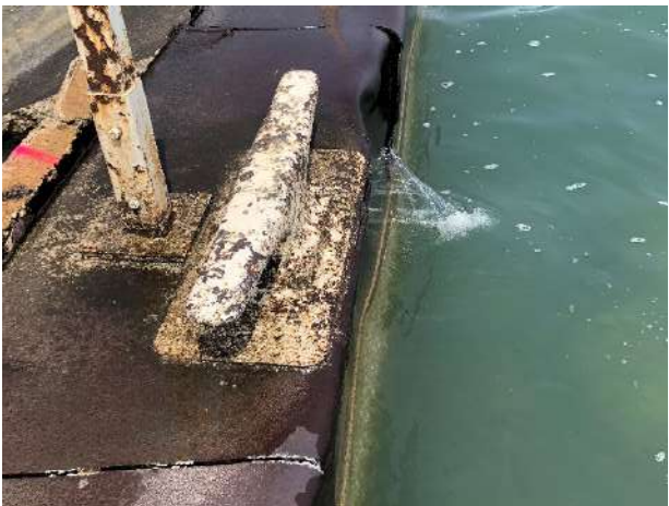
E. Water Escaping through Cracks in Box
