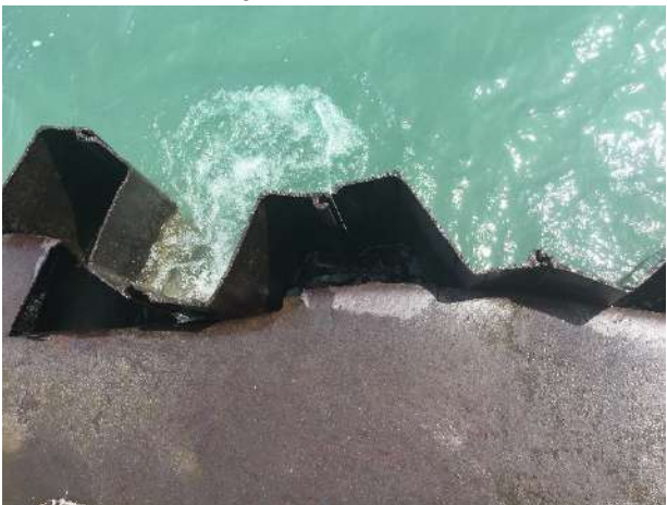
C. Bent/Broken Sheetpile Connections & Box
