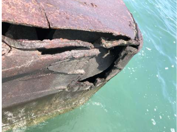
B. Damage to SE Outside Corner
