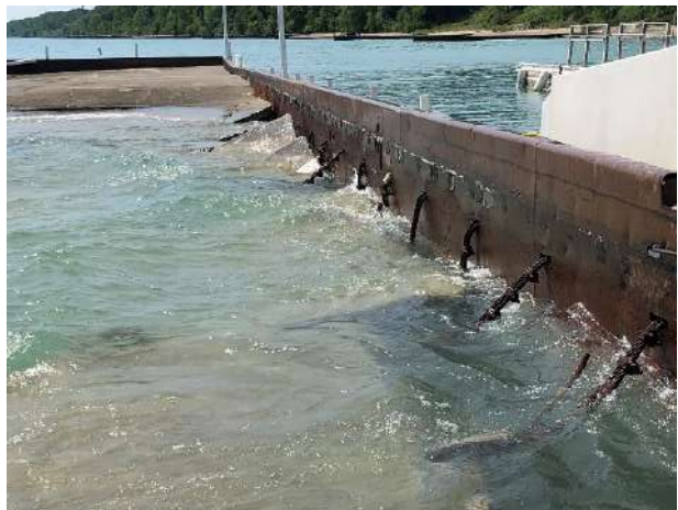
F. Broken Wire Rope Supports
