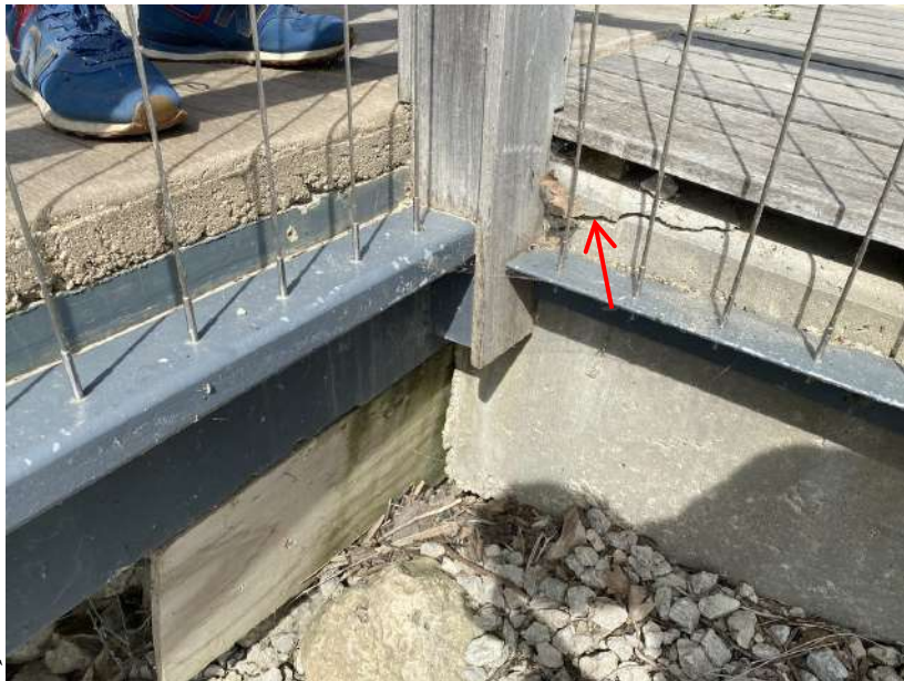
Photo 12 – Crack in Boardwalk Concrete Slab Directly Next to Bridge
