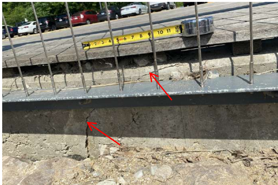
Photo 11 – Stress Crack in Concrete Slab Approximately 11 feet From Bridge.
