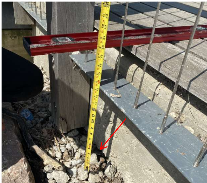
Figure 13 – Downturned (Exposed) Edge of Concrete Slab
